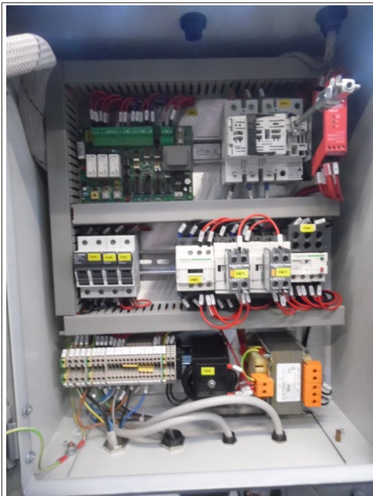
Figure 6-2 – Electric switchboard internal view (Current supply)
